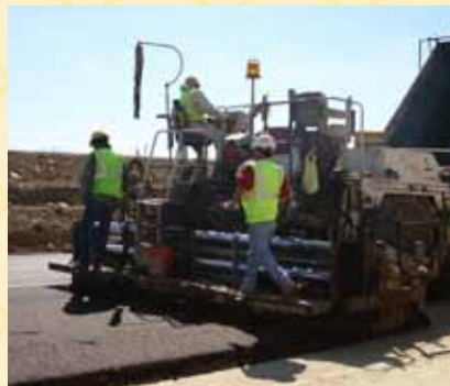
An Austin asphalt crew follows behind as paver places Hotmix on subgrade, preparing the asphalt for the rollers on SH 121.
