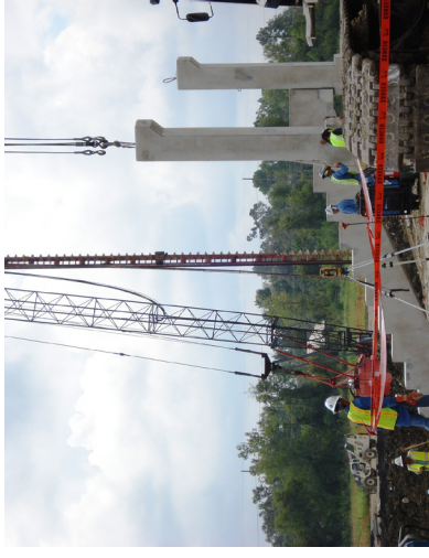
Hallmark Group / Turner Construction JV crew members install precast for the lower level of the stadium
